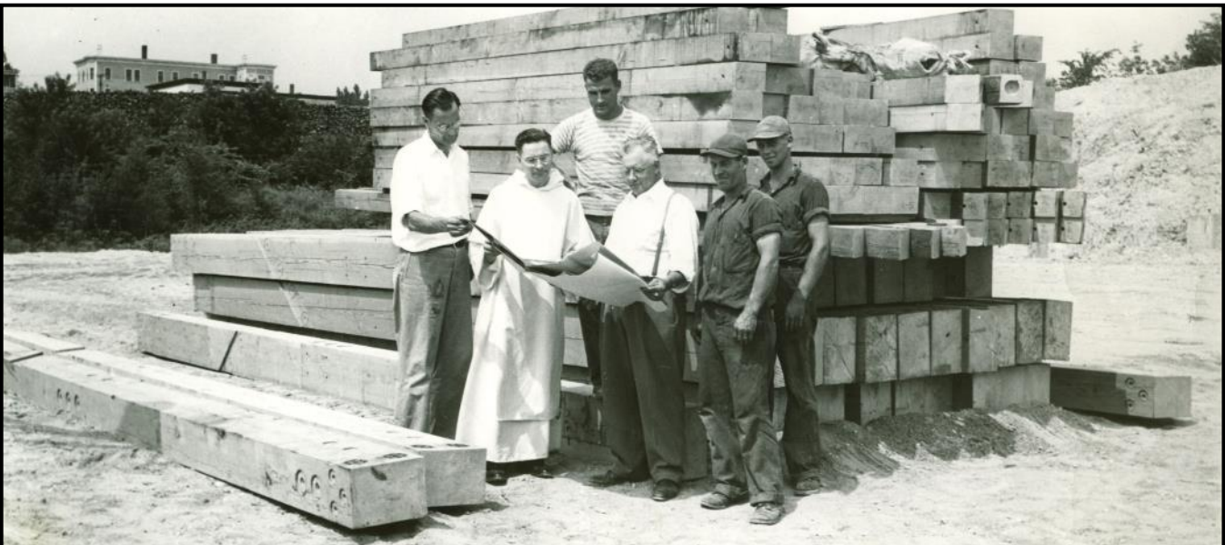
Construction, St Dominic Hockey Arena, Lewiston, c.1949. Fr. François Drouin and Reginald Cloutier discuss the plans for the new indoor arena.
