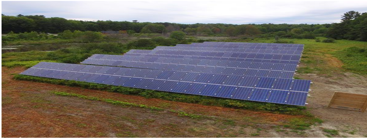
Aerial view of the Maine Idyll Court Community Solar Farm in Freeport, Maine.
